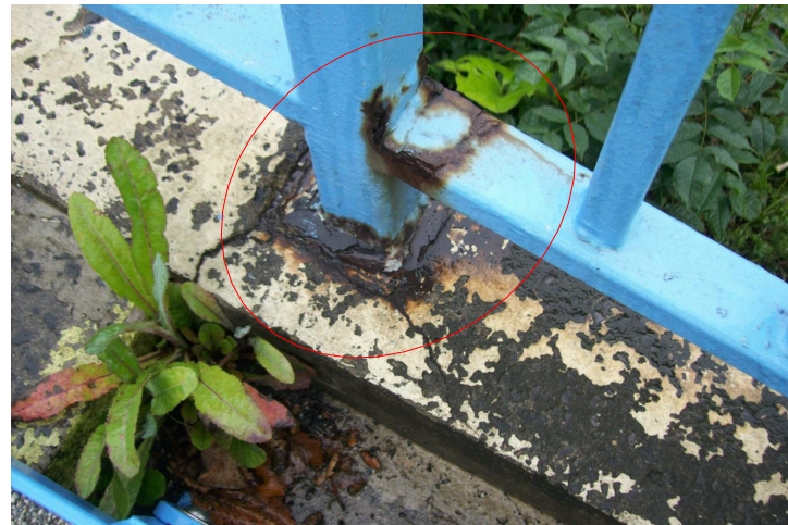
Photograph 1 Typical corrosion to parapet elements across the ramp
