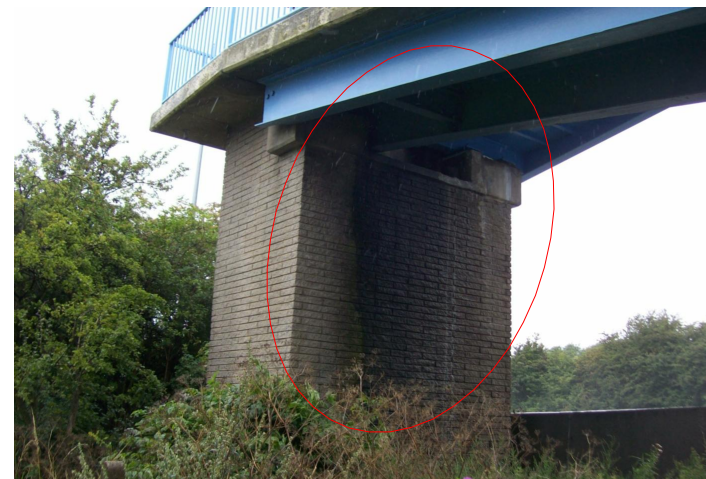
Photograph 2 Staining due to water leakage
